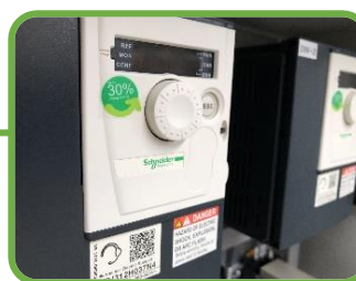
Inverter controller for Screw shafts and Mixing agitator speed adjusting.
